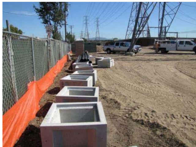
Catch basins, now underground, line the perimeter of the property to ensure that water does not run off site. Bioswales, percolation trenches and five detention chambers provide primary protection against
