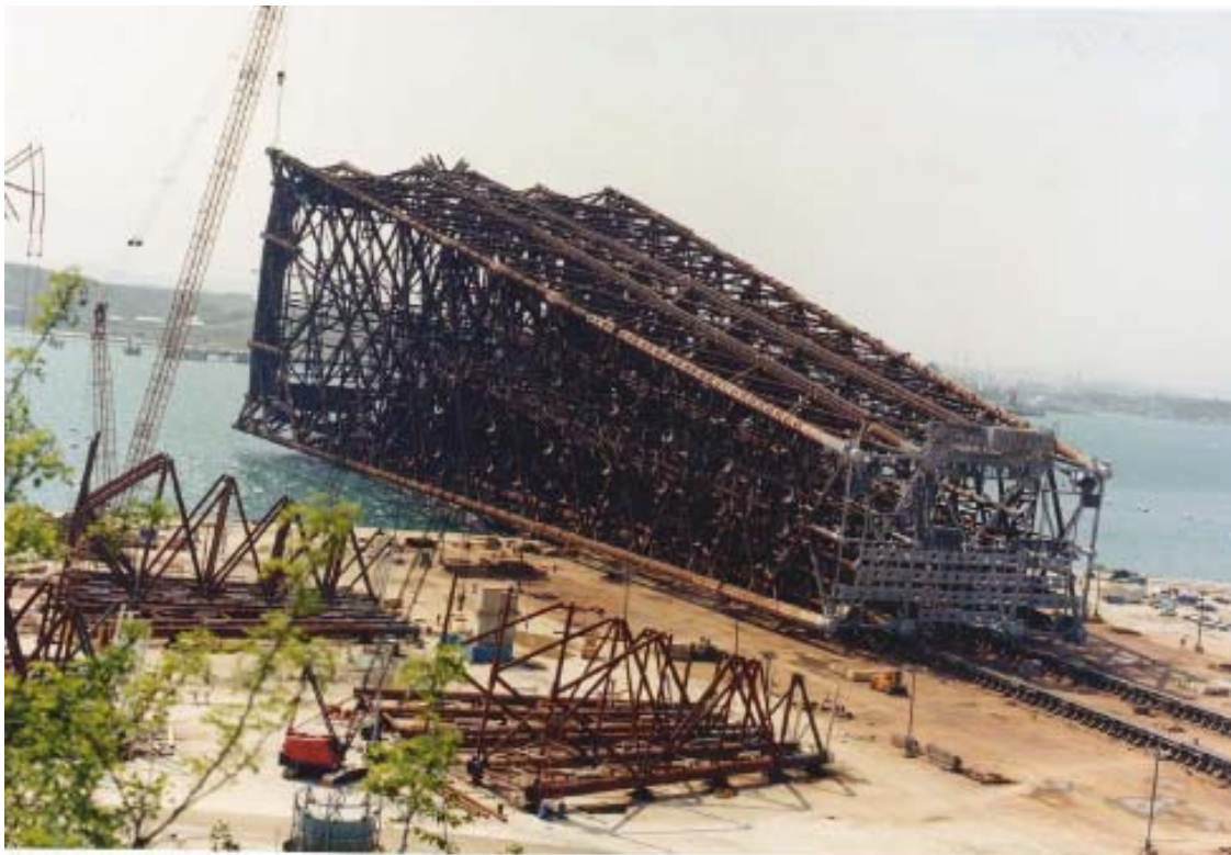
Figure ES.2. A segment of one of the larger California platforms onshore prior to its installation. For scale, a large red crane is in the foreground and a number of trucks and other vehicles are on the shoreline behind the platform at the right edge of the picture (courtesy of Proserv Offshore, Inc.)
