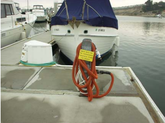
Dunes Marina, inoperable pumpout station. 7/1/02
