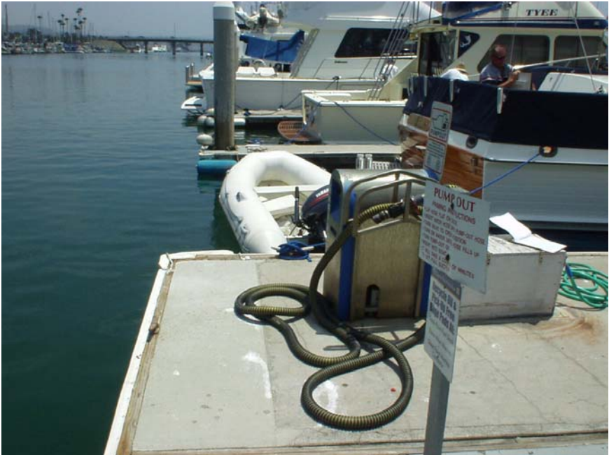
Photo Taken 7/15/02. Dana Point Harbor End of “F” Dock pumpout station.
